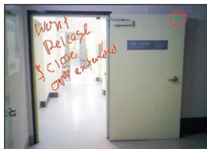
BCA Fire Audit – fire isolated stair Defect – Fire door “won’t release & close as the arm is over extended”
