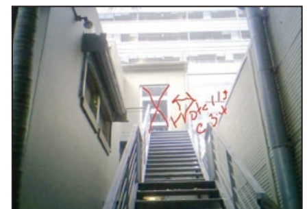
BCA Fire Audit – external building second egress door within 3m of boundary Defect – “Opening not protected as per C3.4 BCA”
